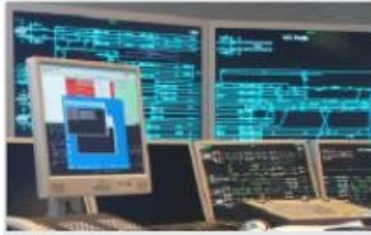
EBI Screen control room
