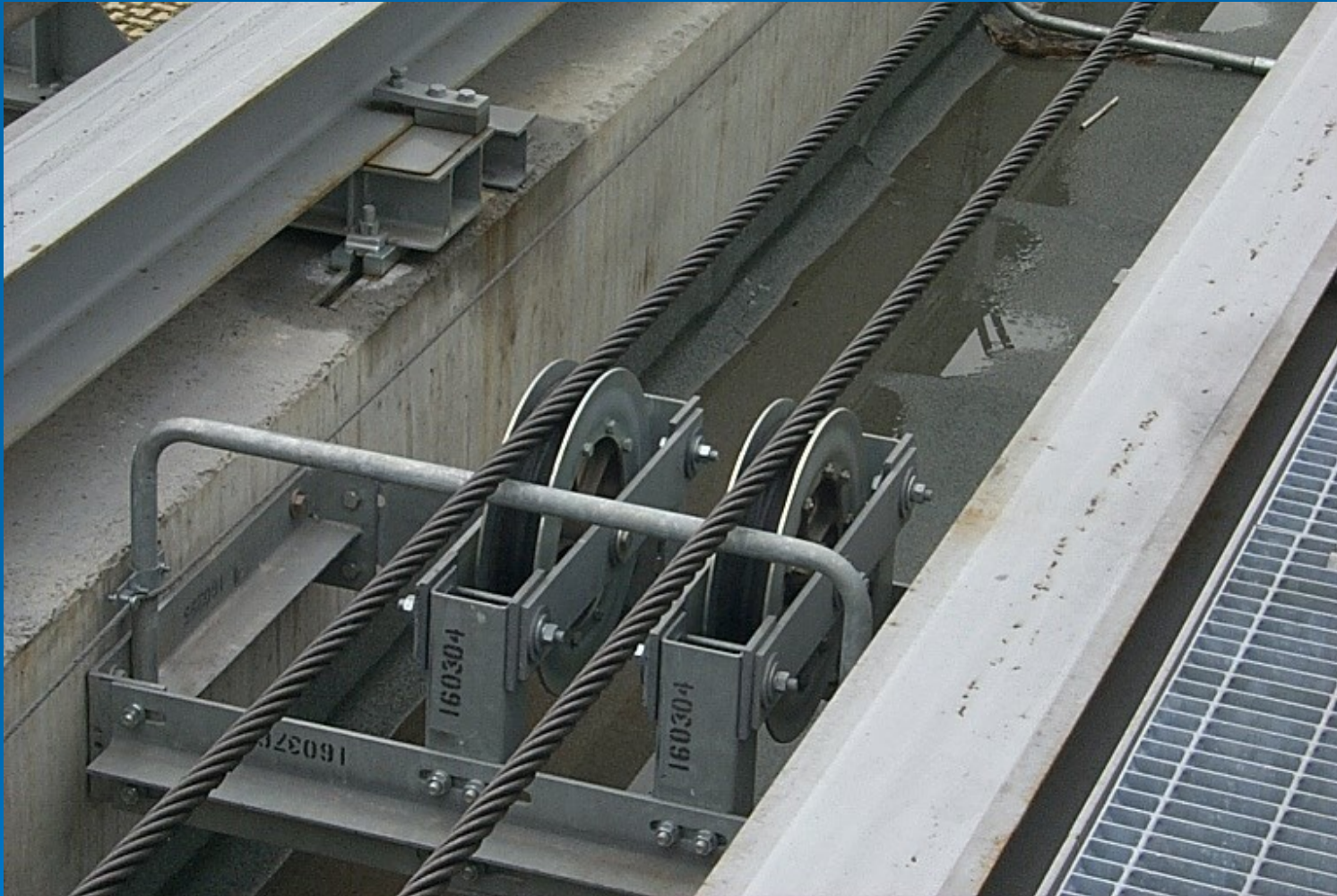
Vertical rollers and anti-derailment system along the line.
